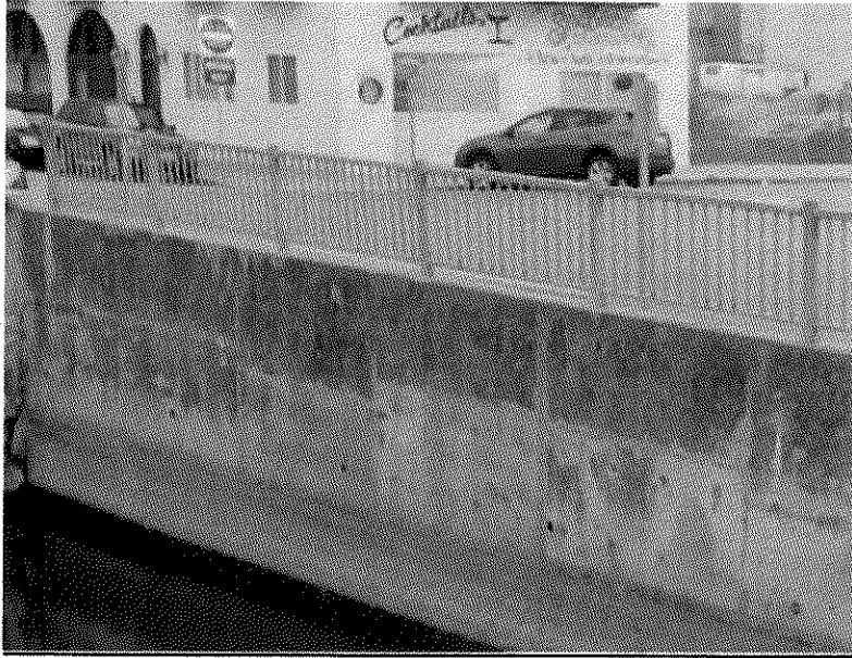
Galvanized Steel Railing on Upper Level of the Vaults (Similar in character to the railing along Aptos Creek)
