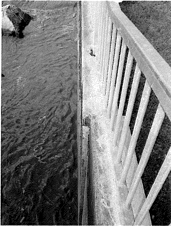
Figure 9: The present-day offset (~2") and tilt in the channel wall immediately adjacent to the State Park's footbridge and existing outfall pipes indicates progression of structural deterioration since the State Park footbridge was built/rebuilt in 1981/1983. Less apparent in the photo angle is evidence of settling offset.
