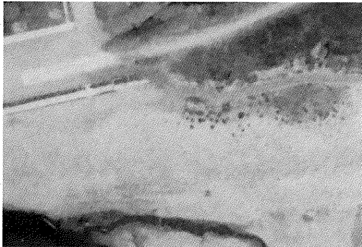
Figure 1: June 1928 photo, taken during a mid-point in extended subdivision construction, indicates that the chosen point for the proposed out-fall location has, comparative to the performance history of the actually developed creek outfall location, become a stabilized area. This is in evidence by the quickly established vegetated tops of sand dunes seen on the back-beach once Aptos Creek flows were channelized away. Approval and filing of Sub-division #5 was made in June 1926, so the realignment of Aptos Creek had not occurred for longer than two seasons.
