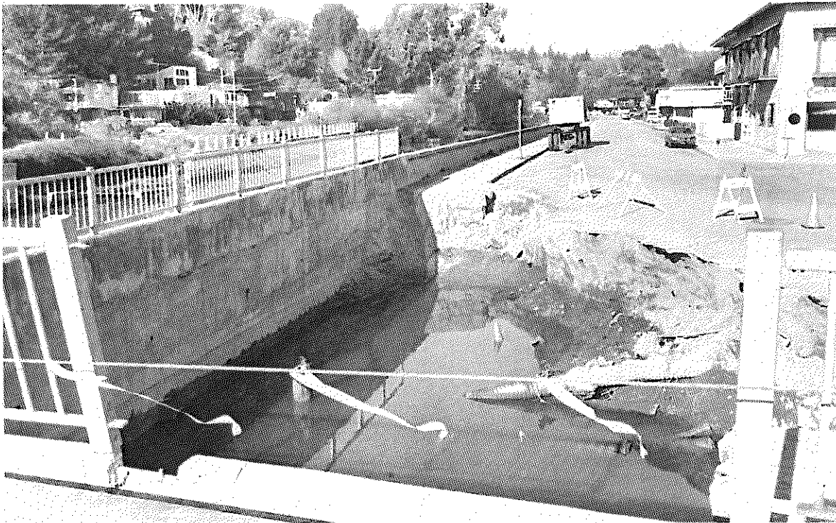
When the rains stopped, there was a gaping hole in the Rio del Mar Esplanade where Aptos Creek runs into Monterey Bay.
