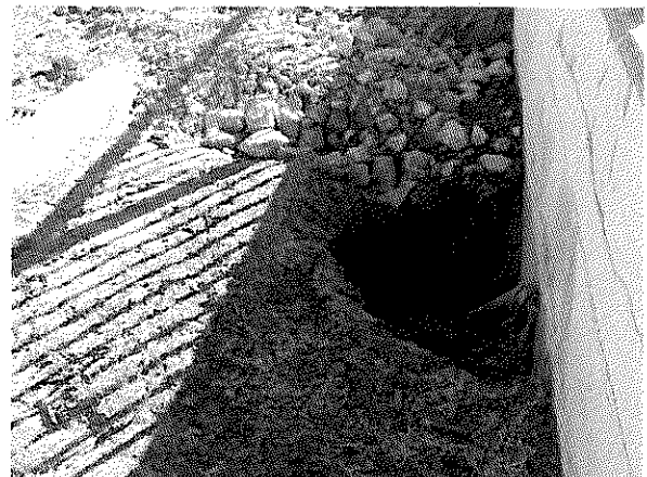
Figure 11: Present-day, multiple sinkholes indicate recurring loss of backfill from behind the cracked channel wall at the same location as much more extensive backfill loss during the 1982 storm. The drainage grate and curb at left edge of photo marks the existing outfall position.
