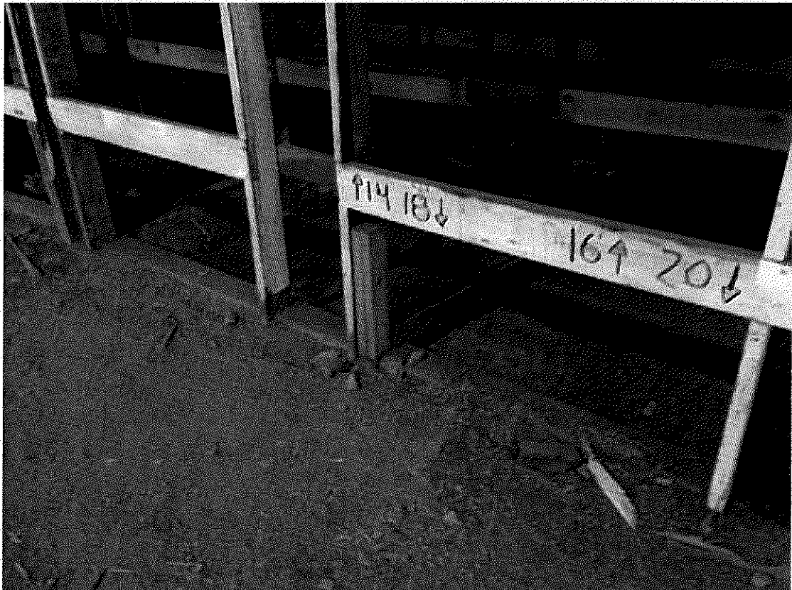
LUMBER STORAGE RACKS CONSTRUCTED ON BARE SOIL
