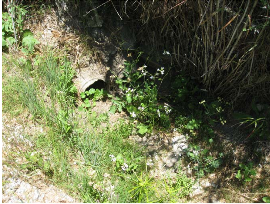
Dual 12" HDPE outlets in vegetated swale
