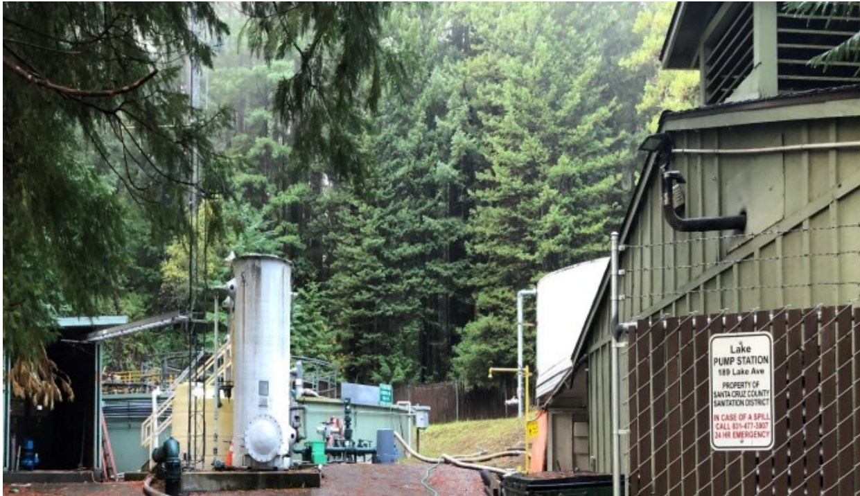
Boulder Creek Treatment Plant Photo Credit: Santa Cruz County
